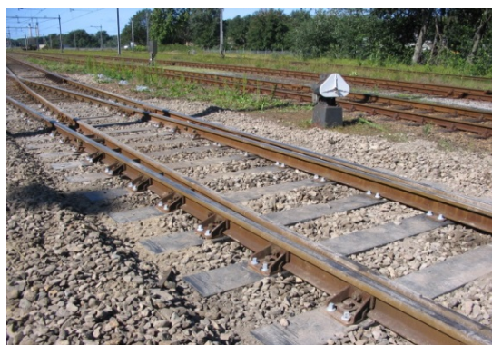
KLP® Hybrid Polymer Turnouts at Corus-Tata Steel, Netherlands
